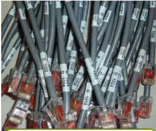
Patch cord labeling
