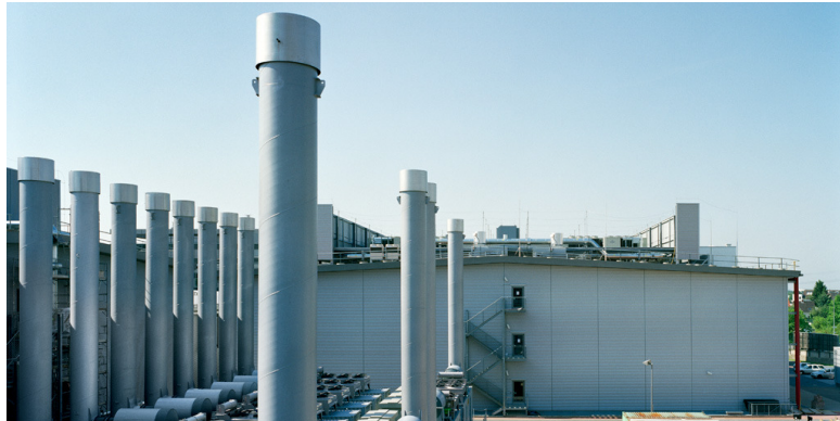
e-shelter Campus Frankfurt 1, Foto
